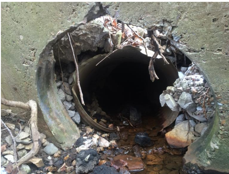
Figure 3: Degraded south end of culvert under Freedom Nissan Parking Lot
