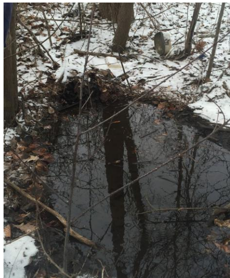
Figure 7: Buried culvert pipe filled with leaves and sediment (Adjacent to the graveyard on the North side of Freedom Nissan)
