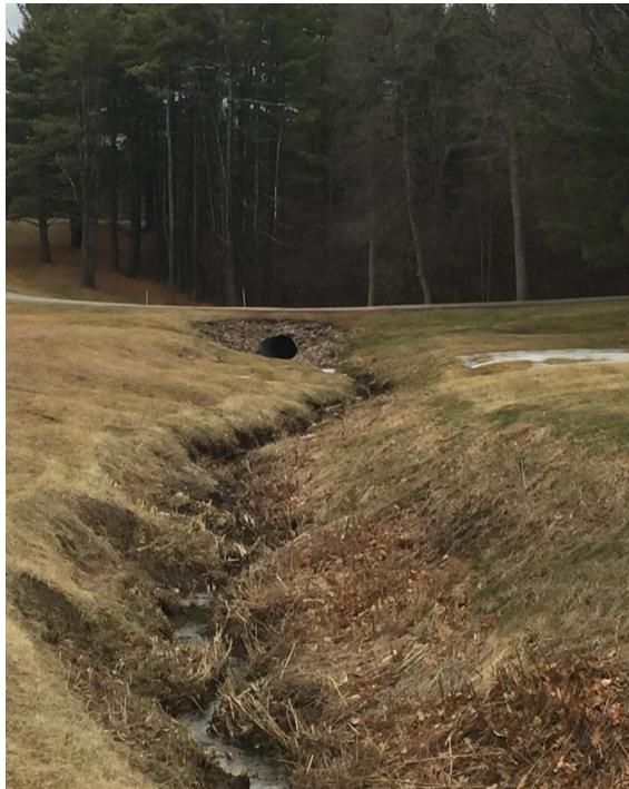
Figure 12: Stream banks below railroad tracks though field
