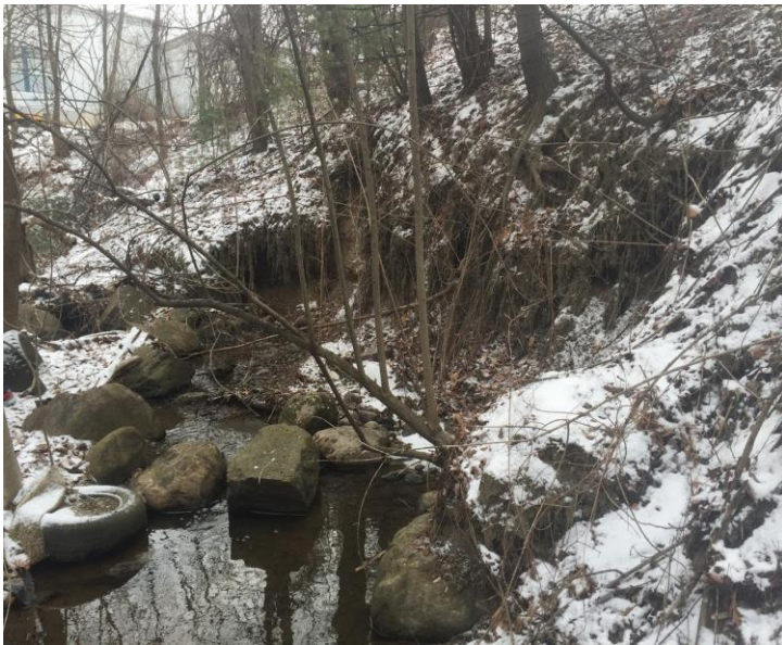
Figure 6: Bank Erosion (South side of Freedom Nissan)
